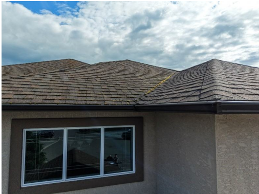
Figure 26. Detail 1 — Roofing Material / Shingle Curl, Multiple.
