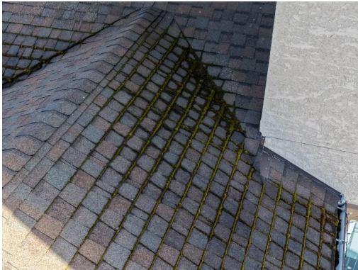
Figure 34. Detail 3 — Moisture Risk / Moss Growth, North.
