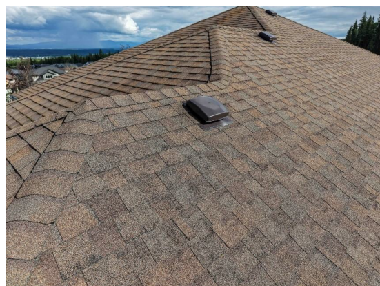
Figure 24. Detail 2 — Roofing Material / Shingle Granule Loss, Multiple.
