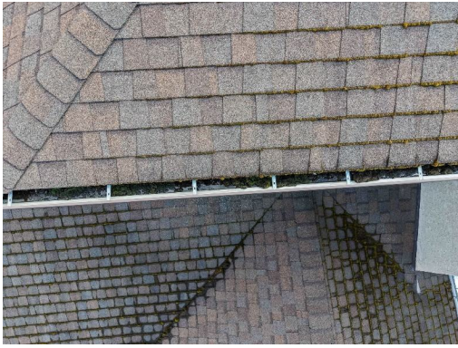
Figure 32. Detail 1 — Moisture Risk / Moss Growth, North.
