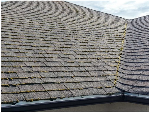
Figure 28. Detail 3 — Roofing Material / Shingle Curl, Multiple.
