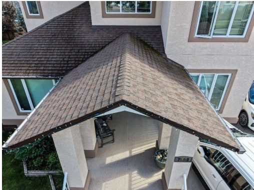
Figure 27. Detail 2 — Roofing Material / Shingle Curl, Multiple.
