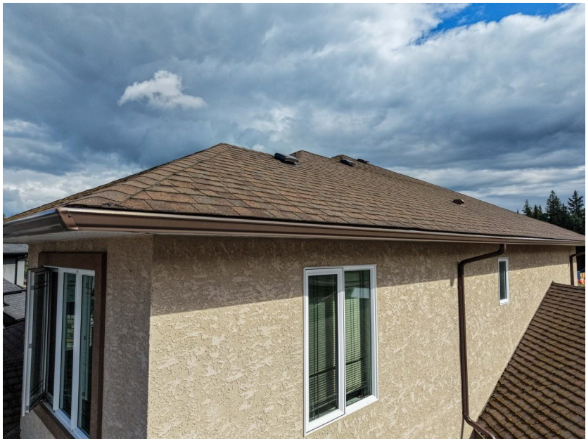
Figure 25. Overview — Roofing Material / Shingle Curl, Multiple.
