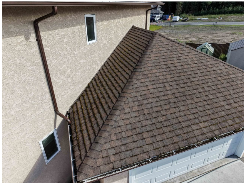
Figure 22. Overview — Roofing Material / Shingle Granule Loss, Multiple.
