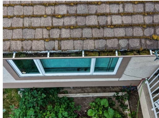
Figure 35. Detail 4 — Moisture Risk / Moss Growth, North.
