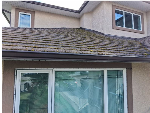
Figure 30. Detail 5 — Roofing Material / Shingle Curl, Multiple.
