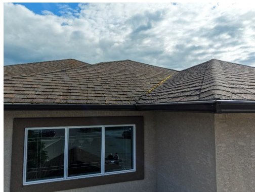
Figure 36. Detail 5 — Moisture Risk / Moss Growth, North.
