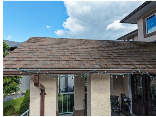
Figure 29. Detail 4 — Roofing Material / Shingle Curl, Multiple.
